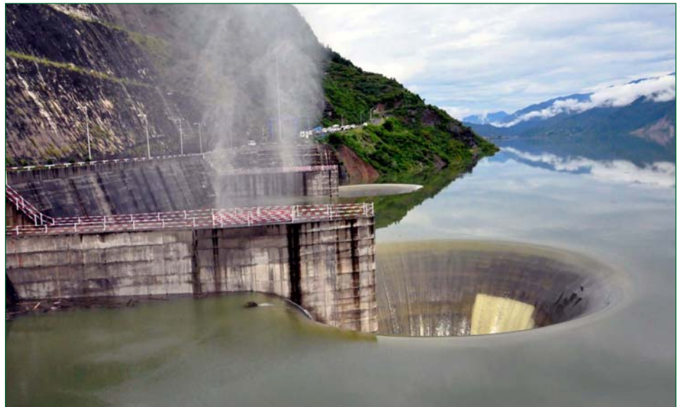
Tehri Right Bank Shaft Spillway (Morning Glory) in operation evacuating floods above the Full Reservoir Level
