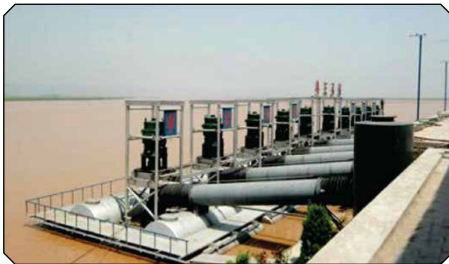
Floating pumping station on Yellow River
