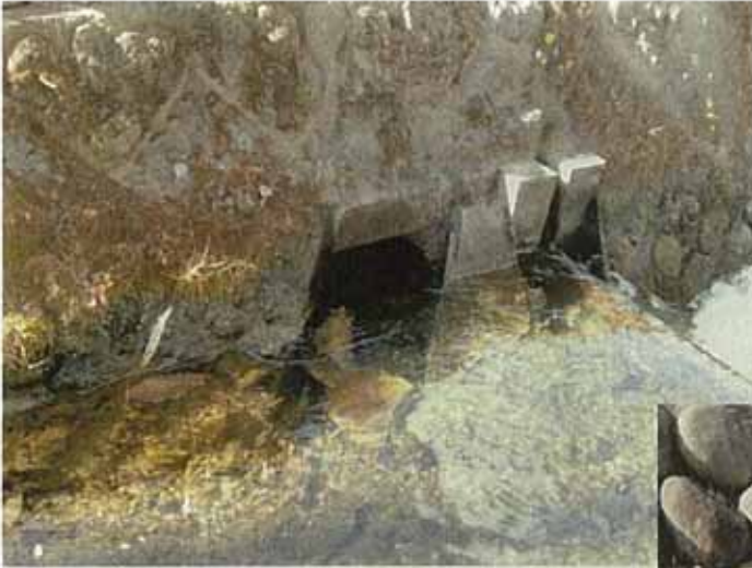
Water intake in main canal (Ichiban-guchi)
