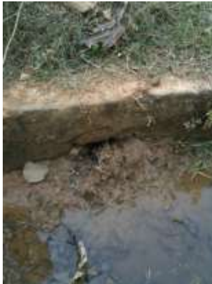
(a) Ungated pipe outlet closed off with mud
