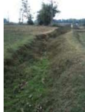
(d) Unlined canal section at tail of the same system. No uniform shape, high seepage losses and unable to maintain command at outlets, OCTMP, Odisha.
