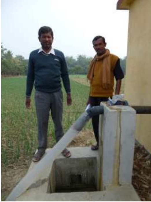
(a) Outlet from the tubewell with the flow meter located in the pipe at the top of the concrete pillar, Shikara-I LDTW irrigation scheme, West Bengal
