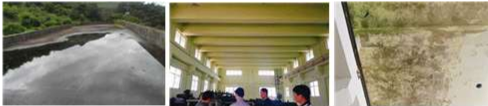
Figure 6. Roof ponding, Flat Roof and Paint Peeling on ceiling
