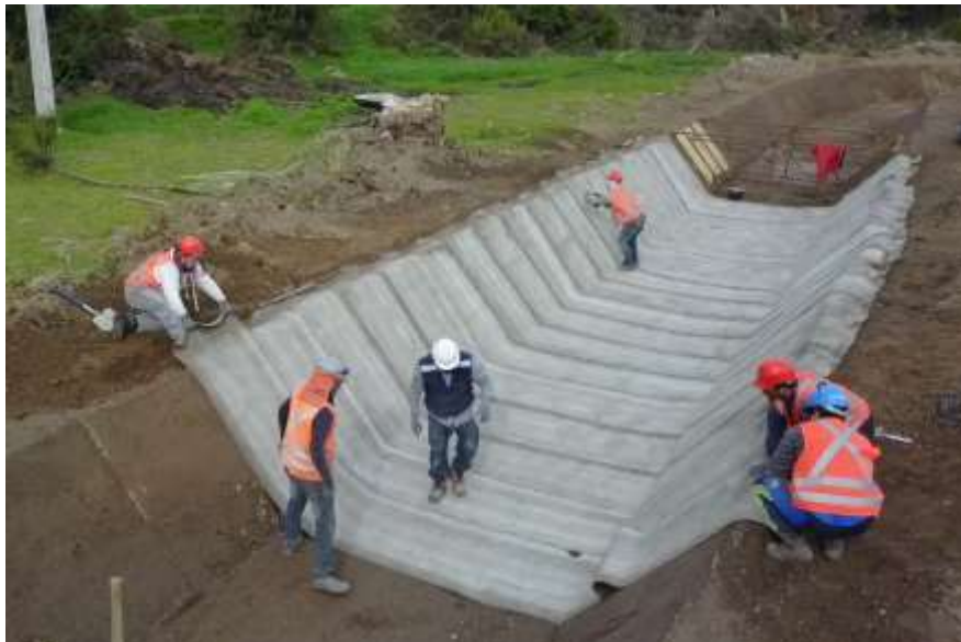
Figure 2. GCCM on the Bella Vista Irrigation Channel. Compaction formwork shown in background.
