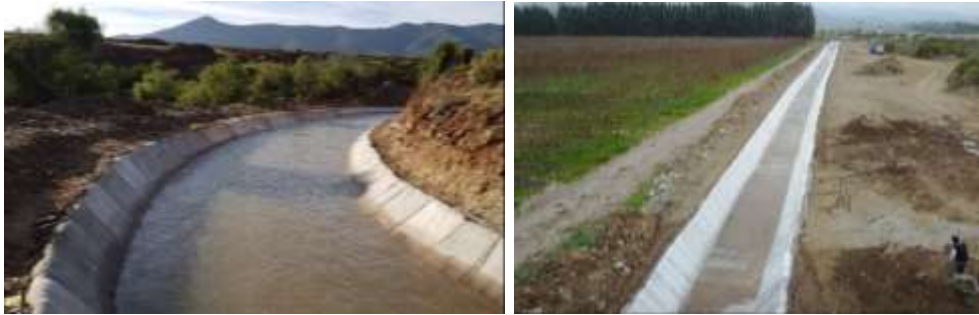
Figure 3. Sections of complete installation prior and during service.
