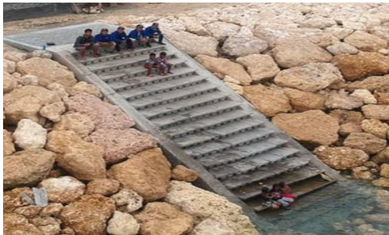
Figure 4. Modular Revetment for Beach Protection (source :Pusair, 2018)
