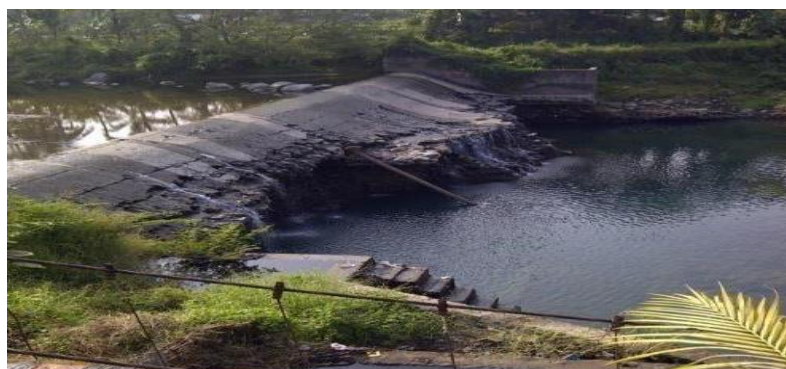
Figure 6. Weir Structure Failure (source :Pusair, 2017)
